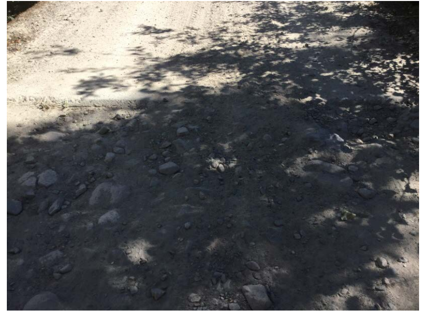
Potholes left approach
